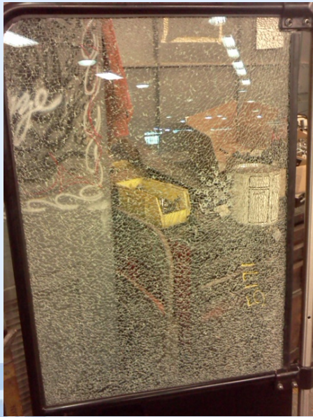
Glass broke because of stress created at upper hinge area
